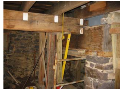
Kitchen summer beam reinforced with inserted channel-beam and fiber glass rods and reset on kitchen fireplace lintel
