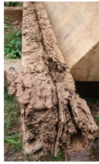
Severely termite damaged kitchen summer beam
