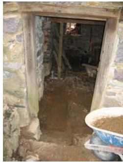
Ground level kitchen doorway 19th century millstone stoop 18th century stone door-sill
